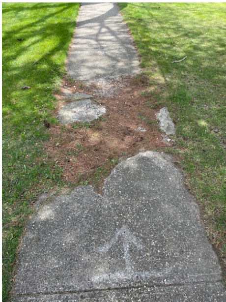
Sidewalk condition issue on Adams St
