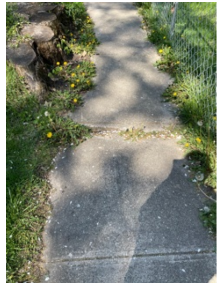
Vertical faults and vegetation overgrowth along Monroe St
