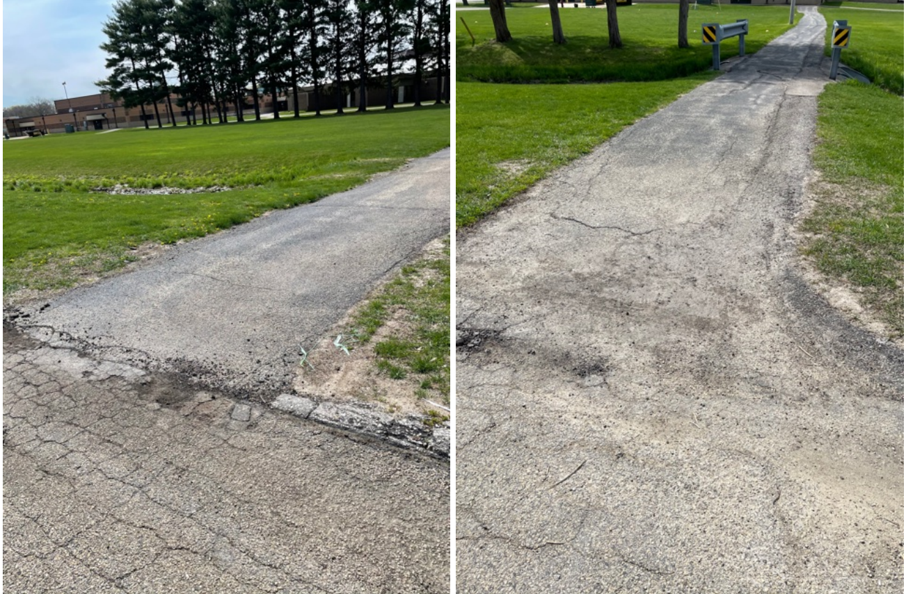
School walkways and Koontz Pl intersections lacking flush transitions and ADA detectable warning strips
